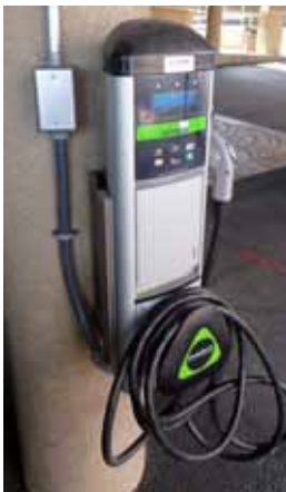
Charging station at the Holiday Inn Express
